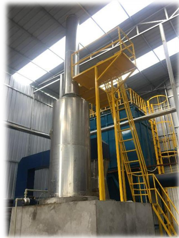
脱硫塔 Desulfurization Tower
