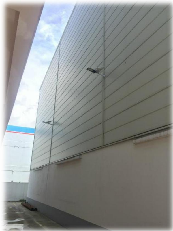
已安装27支太阳能路灯 27 sets solar lighting is running
