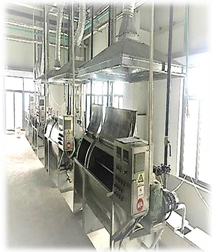
染色工场气过滤系统 Air Filtration System in dyeing workshop
