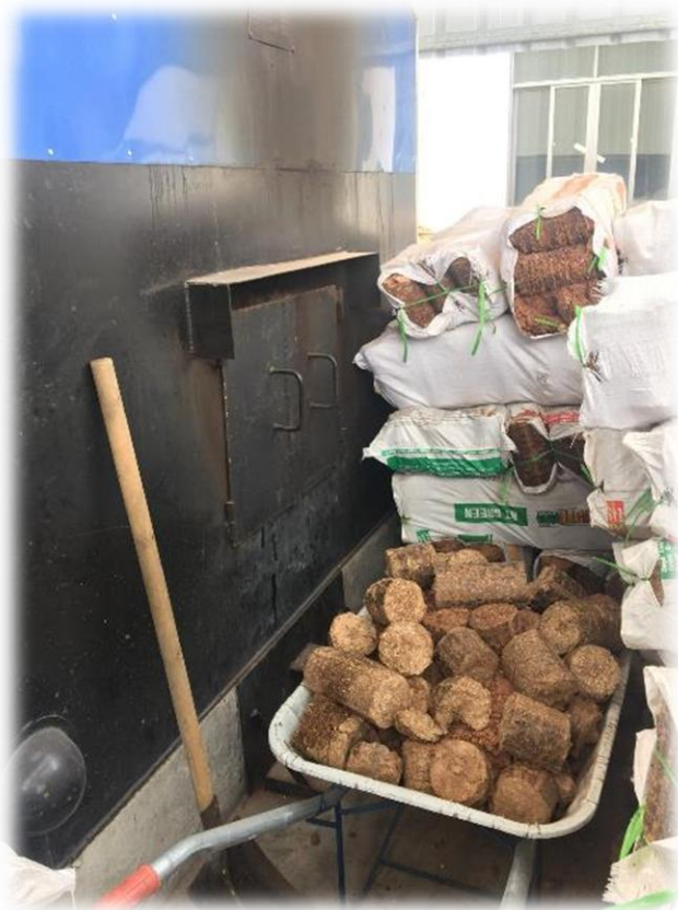
生物质燃料 Boiler is used biomass
